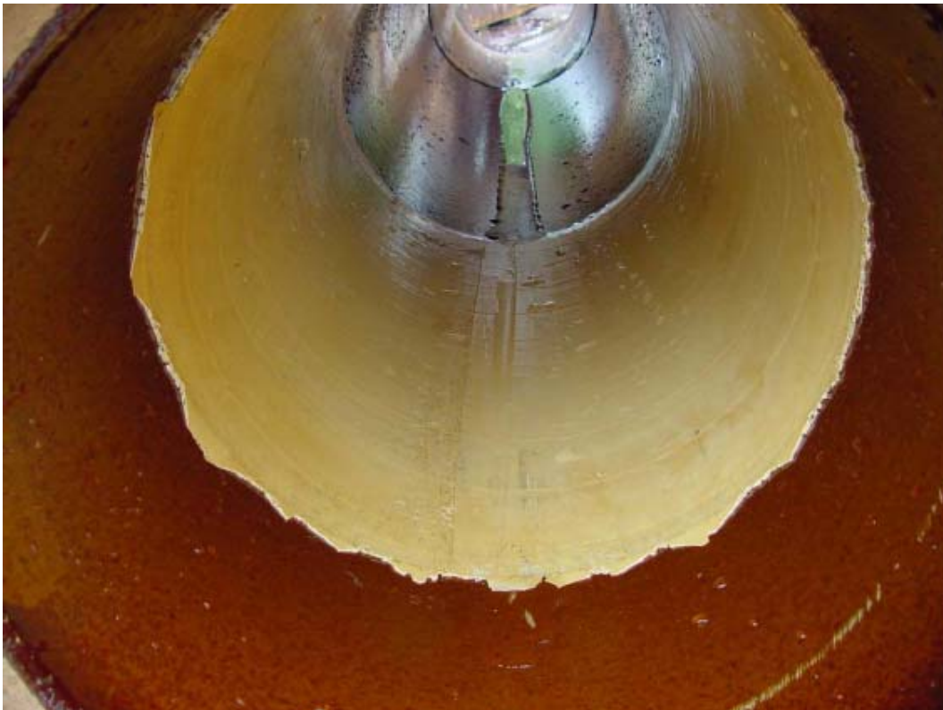
Picture 7: epros patch liner H1263-2.2 after completion of 30 jetter cycles at 80 bar
