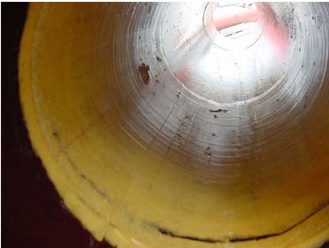
Picture 10: epros patch liner H1263-1.1 after completion of 30 jetter cycles at 80 bar and after stationary load (3 minutes)
