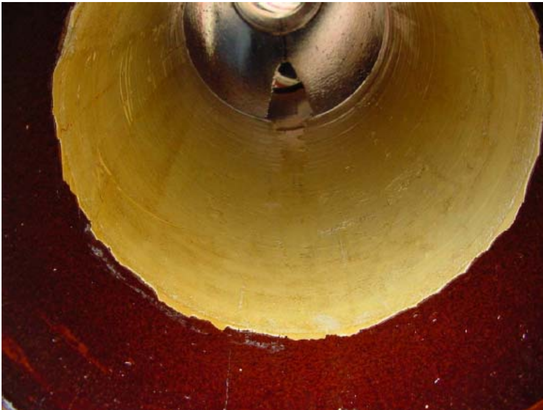
Picture 9: epros patch liner H1263-1.2 after completion of 30 jetter cycles at 80 bar and after stationary load (3 minutes)
